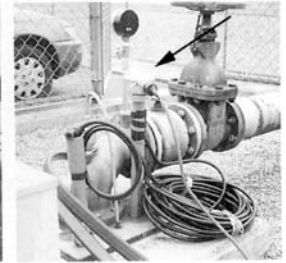
Deep well monitoring with Terminal box
